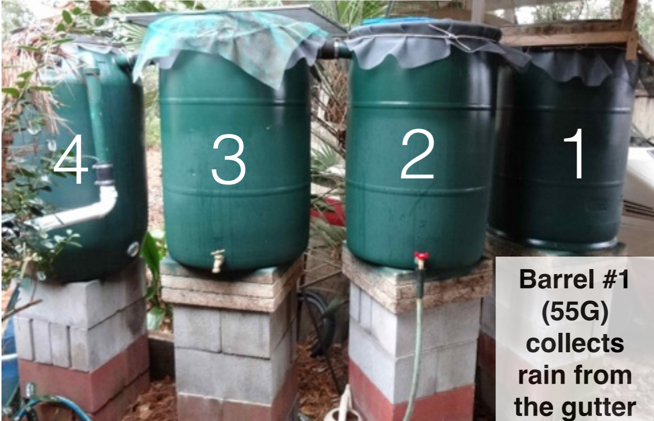
East side: 4 barrels near the house and 2 remote barrels in the garden
