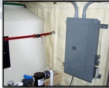
Electric Breaker Panel
