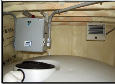
Control Panel & Heater
