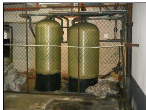
Kirana Residence Domestic Water Tank
