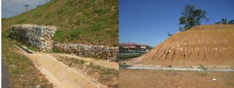
Figure 4. Combination of Geometrical Method with Gabion Wall at the toe of slopes
