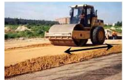
In the field increasing compaction energy = increasing number of passes or reducing lift depth
