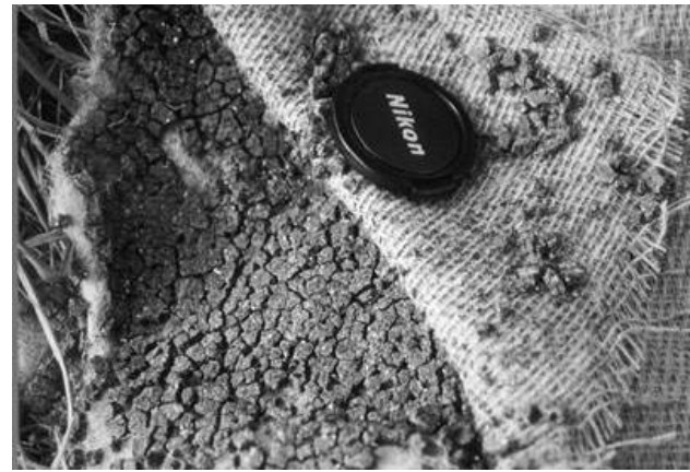
Figure 6. Photograph of desiccated bentonite in a GCL exhumed from a cap in southwestern Wisconsin (from Benson, 2002).
