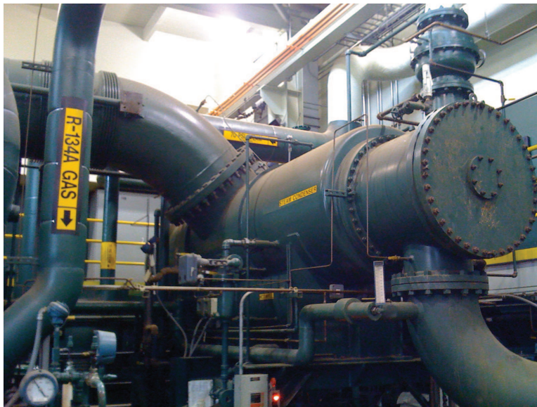
Figure 8.18: Chiller in the University of Notre Dame power plant, 14 June 2010.
