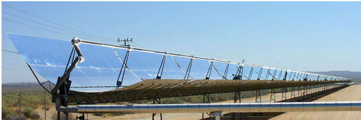
Figure 2.11 Parabolic trough collectors are used to generate electricity in southern California. (credit: “kjkolb”/Wikimedia Commons)
