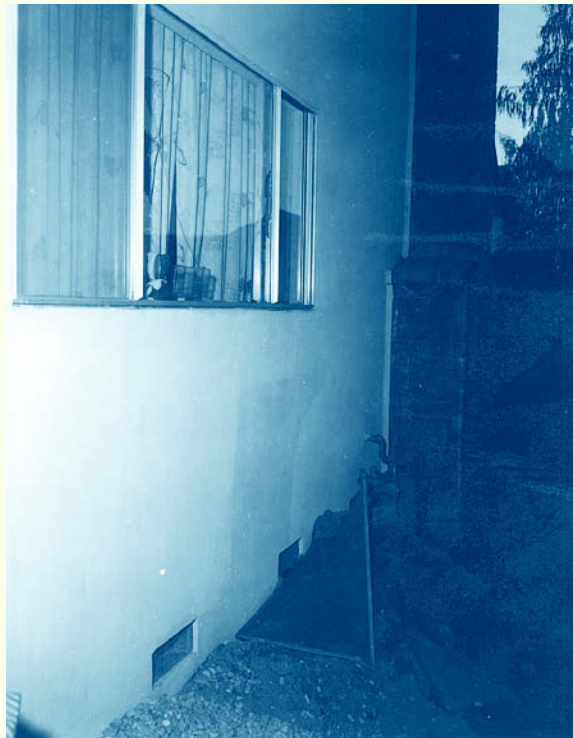
FIGURE 37—The windows in many older buildings were constructed at a height that makes them too easily accessible from the ground.
