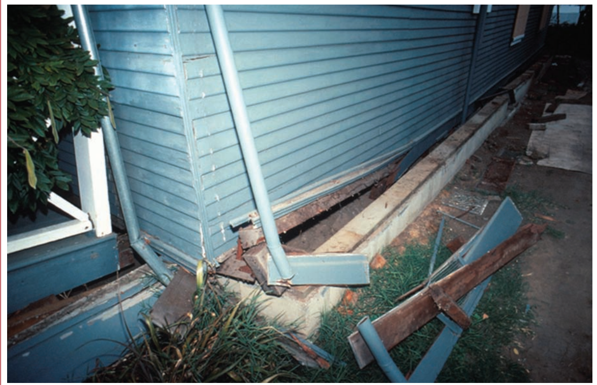
Figure 17 Houses in Watsonville, California, that fell off their foundations in the 1989 Loma Prieta earthquake.
