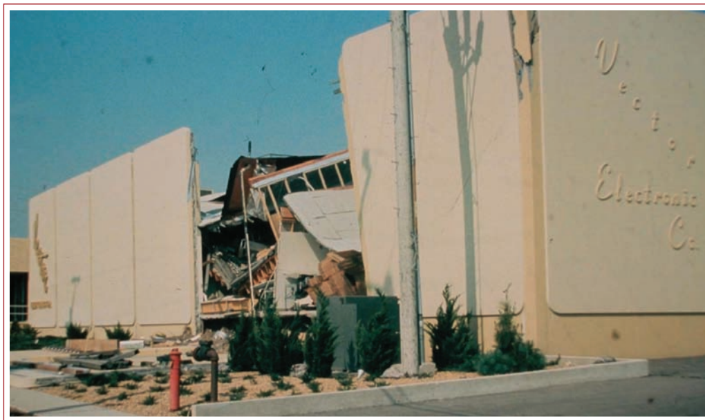
Figure 16 Collapse of a tilt-up building in the 1971 San Fernando earthquake (photo by P. Yaney).
