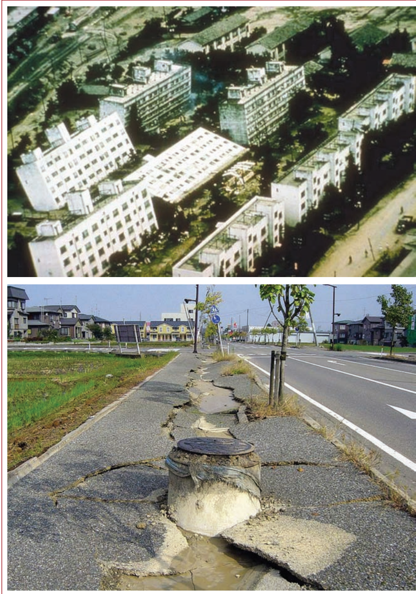
Figure 6 Top photo shows liquefaction-induced settlement of apartment buildings in the 1964 earthquake in Nigata, Japan (photo courtesy of the University of Washington). The bottom photo shows one of many manholes that floated to the surface as a result of soil liquefaction caused by the 2004 Chuetsu earthquake near Nigata, Japan (photo courtesy of Wikimedia Commons).
