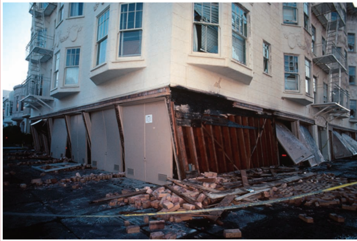
Figure 18 First story of an apartment building in San Francisco, California, leaning to the side after the 1989 Loma Prieta earthquake.
