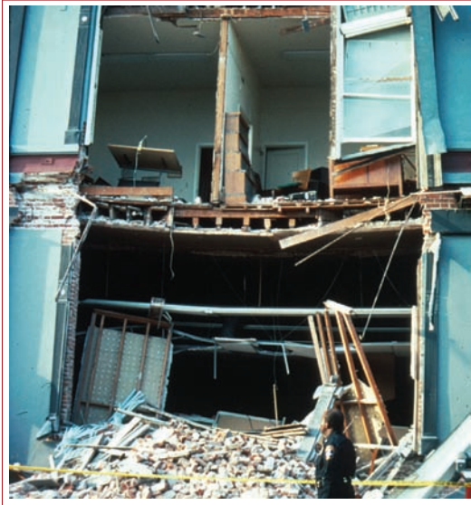
Figure 20 Failure of an unreinforced masonry wall in a building in Santa Cruz, California, in the 1989 Loma Prieta earthquake.
