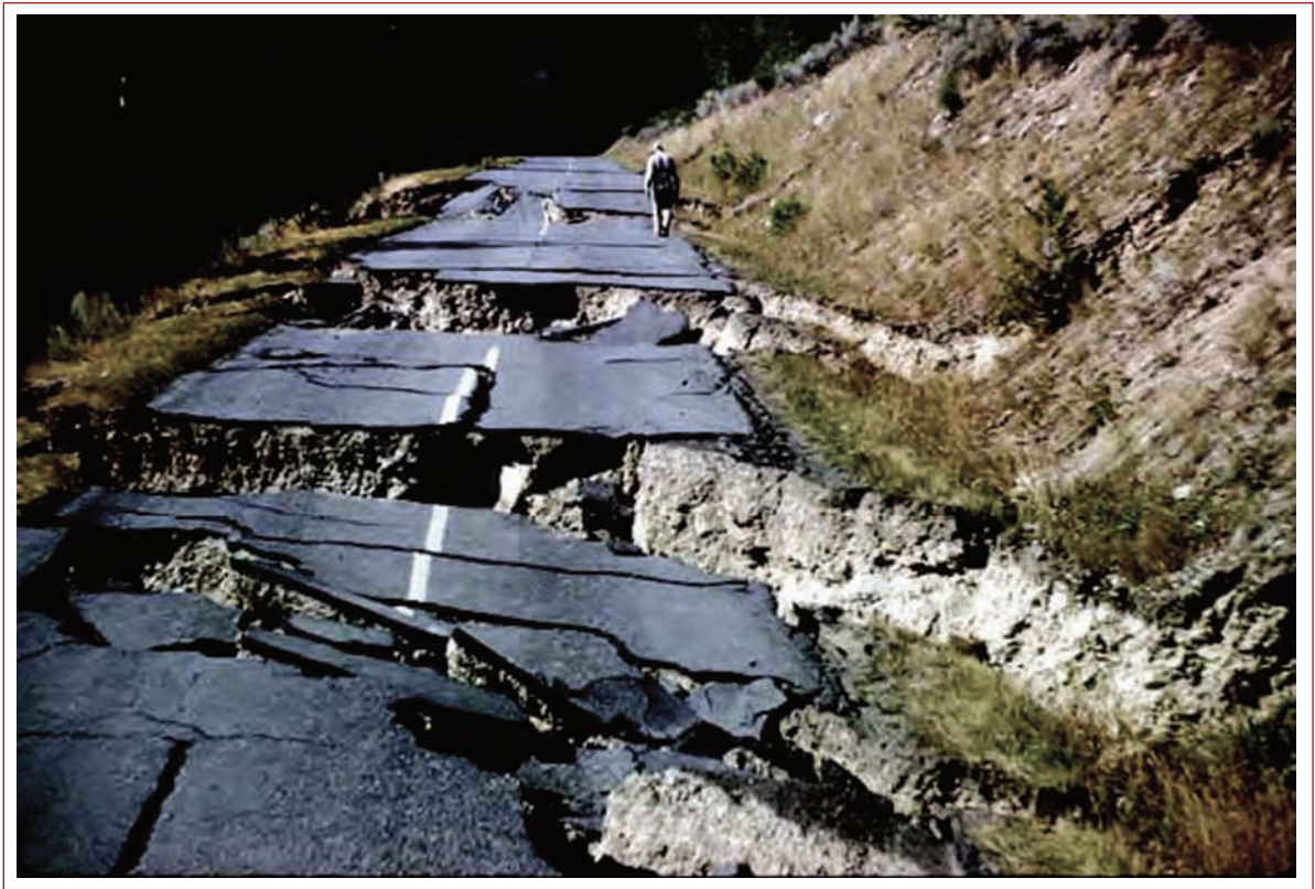
Figure 7 Lateral spreading damage to highway pavement near Yellowstone Park resulting from the 1959 Hegben Lake earthquake (photo courtesy of the USGS).
