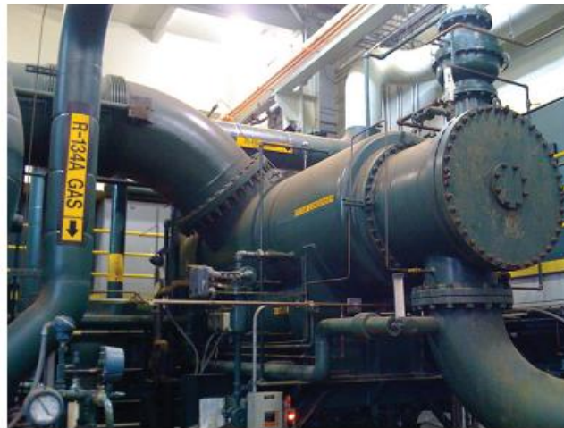
Fig 9.12. Chiller in the University of Notre Dame power plant, 14 June 2010
