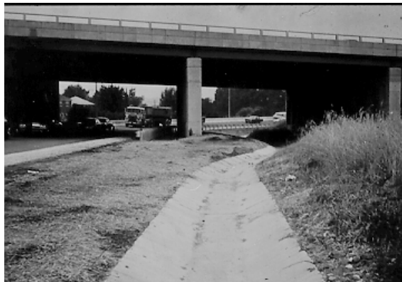
Figure 5.4. Rigid concrete channel lining.
