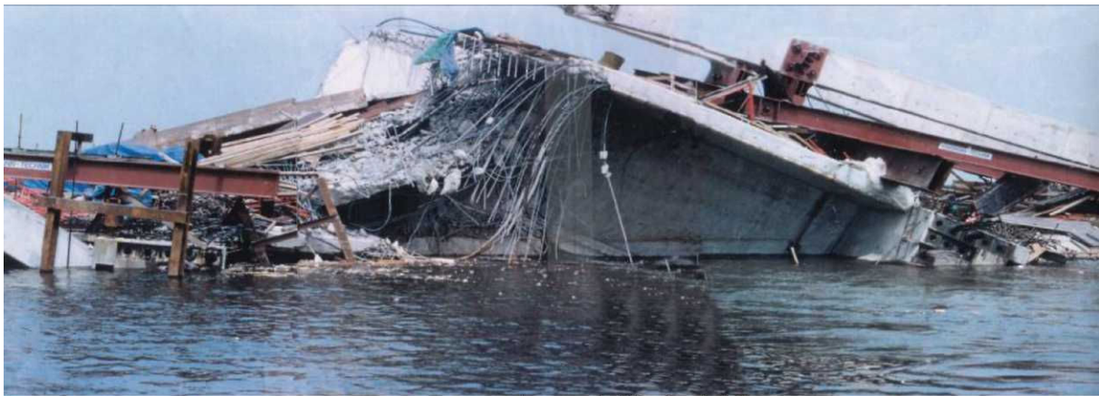
Figure 10 - Collapse of a bridge due to lacking control of the specific ground properties during pile execution (no comparison of design assumptions and locally found soil)
