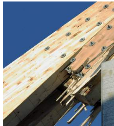
Failed heel joint
