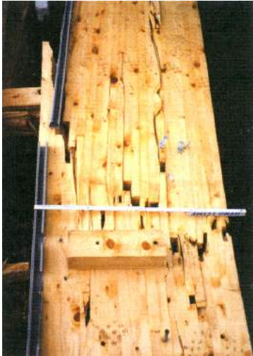
Fig. 10. Failed glulam beam due to low quality finger joints. The failure line is staggered and coincides with the finger joints. Source: Ref. [9].
