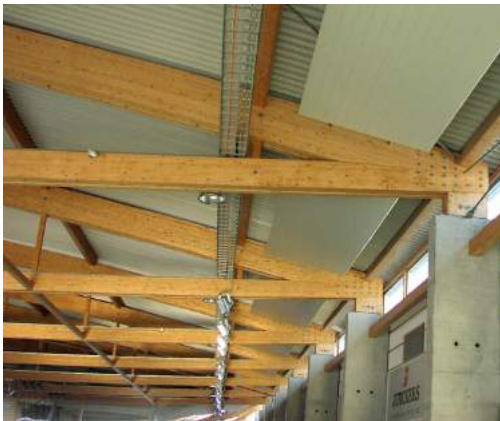
Roof before failure
