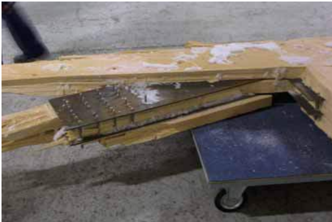
Fig. 3. Slotted-in steel plate joint where dowels were not mounted as intended.
