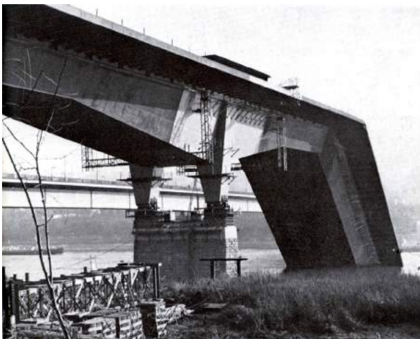
Fig. 8. Collapse of steel box girder during cantilever construction, Rheinbrücke, Koblenz, 1971, Source: Ref. [31].
