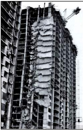
Fig. 4. Progressive failure of multi-storey concrete building due to premature removal of shoring, 1973, Virginia, USA.
