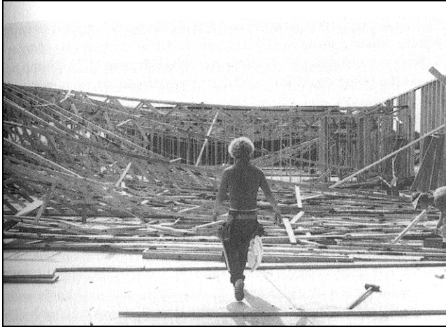
Figure 16. Collapse of timber truss roof during construction. Source: Ref. [33].
