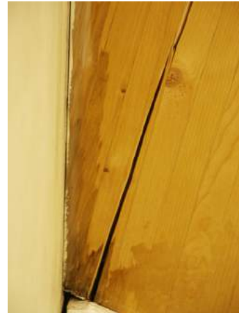
Figure 115-2. Crack at column fitting to the steel part.
