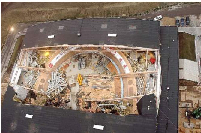
Fig. 2. Photo taken from above after the failure of the Ballerup arena roof.
