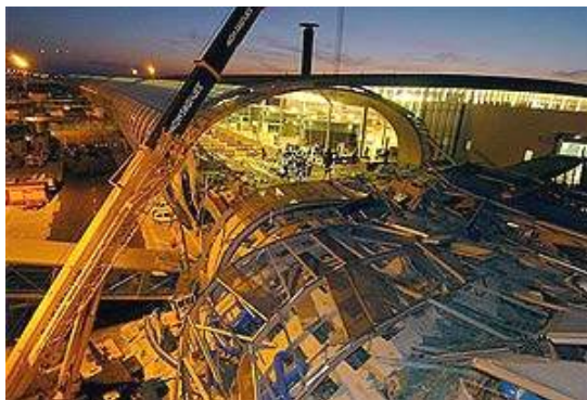
Fig. 6. Collapse of terminal roof at Charles de Gaulle airport in Paris
