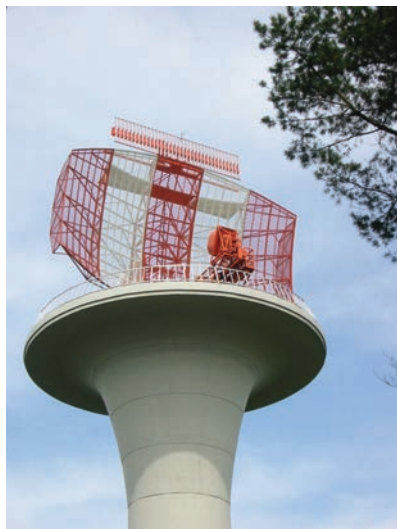
(a) Radar antenna. The parabolic antenna is the PSR and the rectangular one above it is the SSR. © Magnus Manske / Wikimedia Commons / CC-BY-SA-3.0.
