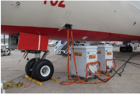
(a) Ground electrical power delivered to a Boeing 787. © Olivier Cleyner / Wikimedia Commons / CC-BY-SA-3.0.
