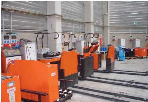
Material stored next to a battery charger (up) and obstacle-free battery-charging area (down)
