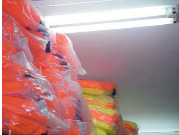
Plastic material stored near lighting
