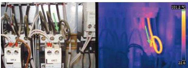
Thermal imaging analysis of a main switchboard. Real image on the left, thermal image on the right.
