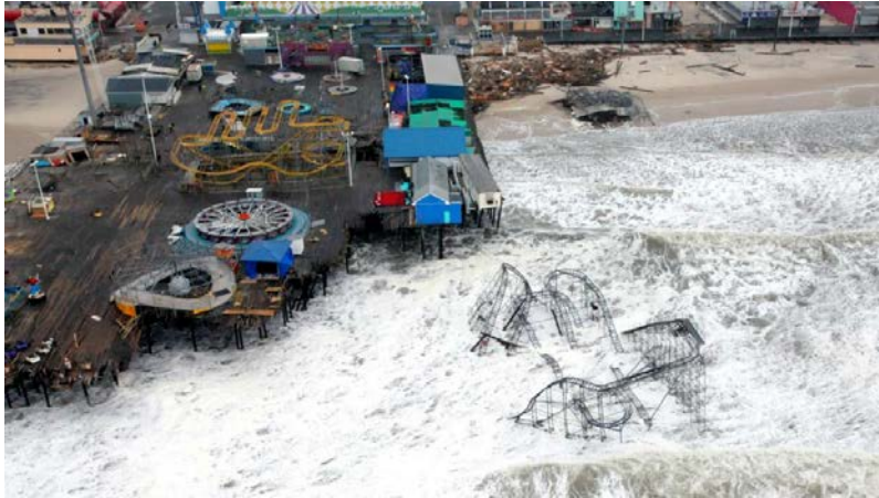
Figure 19.14 Damage to the Casino Pier, Seaside Heights, New Jersey, from Hurricane Sandy, November 2012 [ https://upload.wikimedia.org/wikipedia/commons/c/cb/Hurricane_Sandy_New_Jersey_Pier.jpg ]
