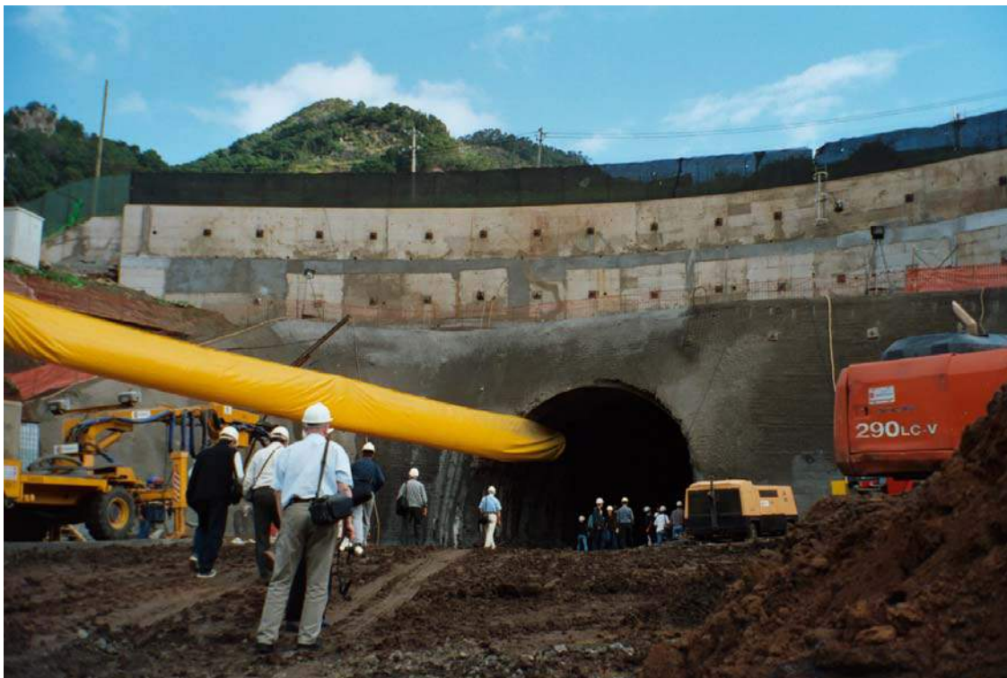
Fig. J-21. Tunnel portal. Note the heavy concrete reinforced and anchored retaining support above the tunnel (Madeira, Portugal)
