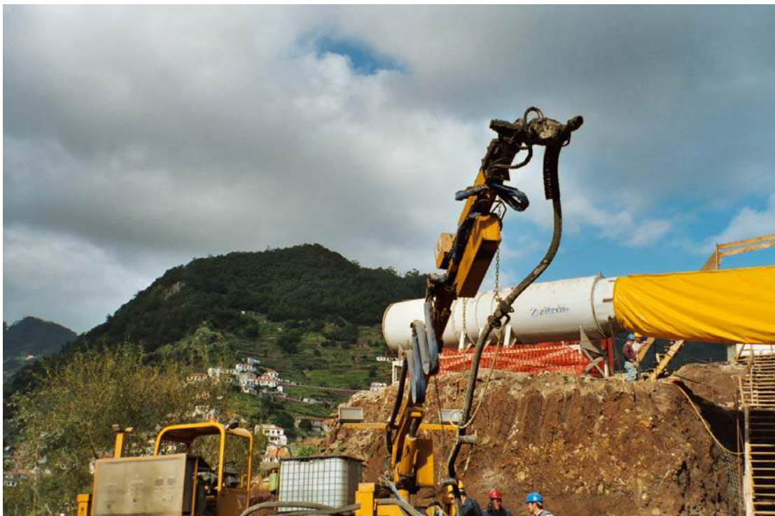
Fig. J-8. Shotcrete nozzle mounted on an arm on a bulldozer (Madeira, Portugal)
