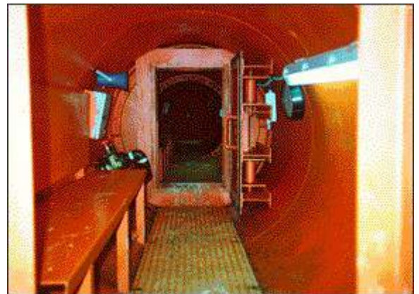
Fig. J-4. Man lock in shield for compressed air tunneling (Singapore Metro: Orchard Road station and tunnel) (photo: Traylor)
