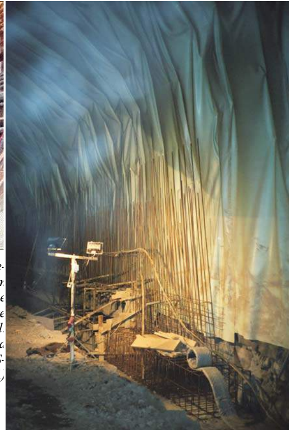
Fig. J-20. Installing reinforcement for poured concrete support. Note the plastic sheeting for diverting water to the sites of the tunnel (Madeira, Portugal)
