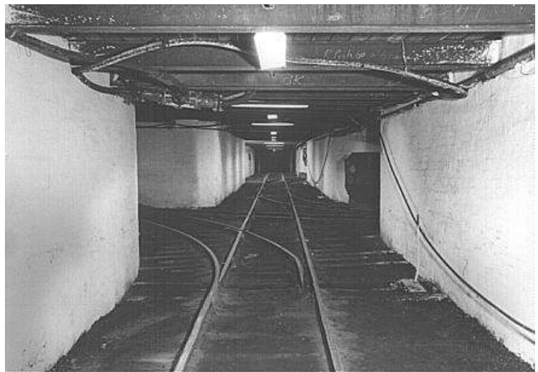
Fig. J-17. Fixed steel beam roof and concrete formed wall support (photo: Underground, Burwood Colliery; Lake Macquarie City Library, Australia )
