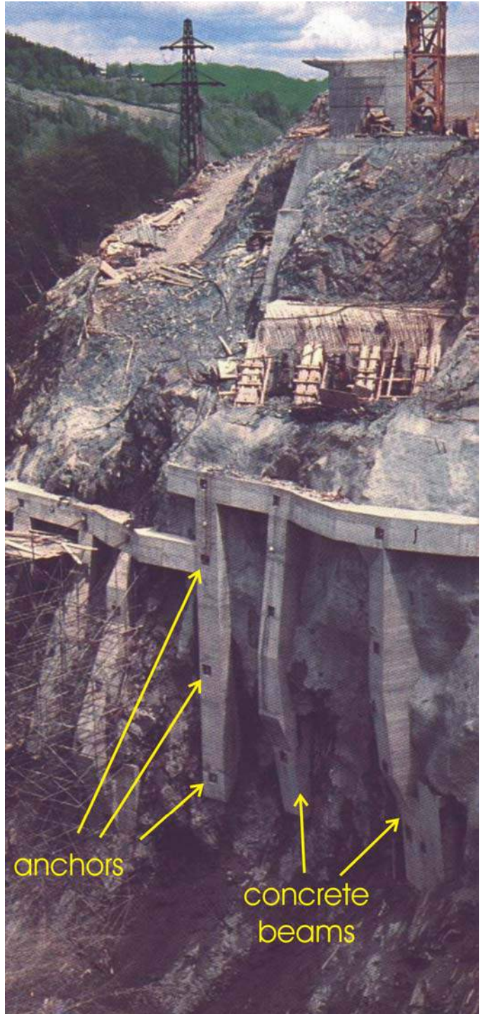
Fig. J-14. Large scale anchoring of the foundations for the abutment of a bridge. Only the anchors plates (small black squares) can be seen on top of reinforced concrete beams (after Geoconsult, Salzburg, 1978)
