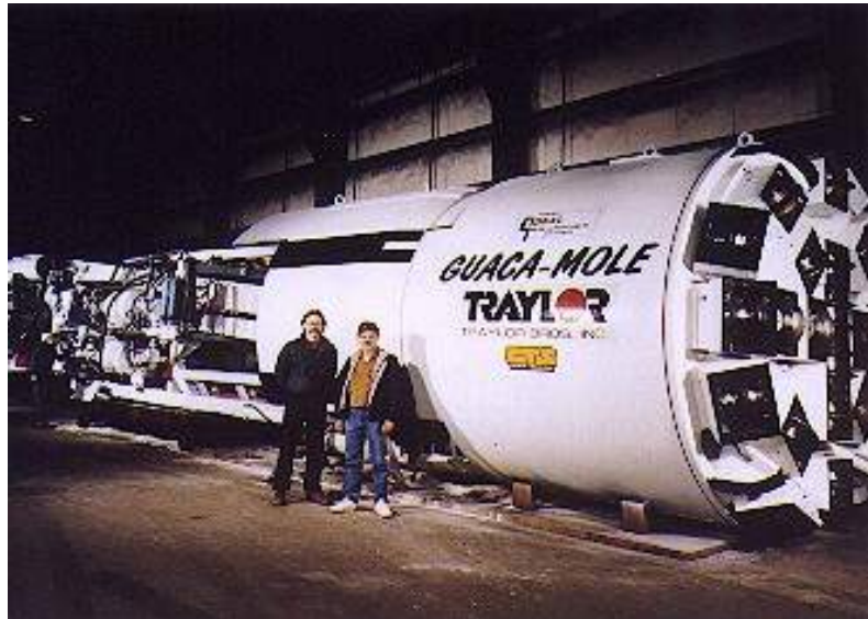
Fig. K-5. TBM with shield used to drill through 413 MPa !! (60,000 psi) granite and a fractured and weathered surface formation, which required immediate support (Cowles Mountain Water Tunnel, San Diego, USA (photo: Traylor)
