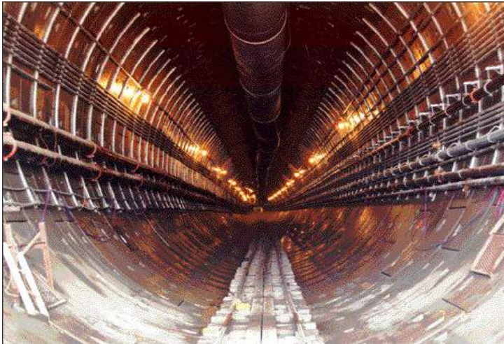
Fig. J-19. Pre-fabricated concrete support. The 10 m (32 ft) diameter EPB tunnel drilled by TBM was excavated with as little as 3.3 m of soft clay between the tunnel and the 21 m deep river bottom. The tunnel approached the river beneath a refinery site, with sensitive laboratory buildings and storage tanks directly over the tunnel. Forces and soil pressures were controlled with computer-monitored sensors. Expected settlements did not occur. (CN Rails's U.S.-Canada Tunnel beneath the St. Clair River at Port Huron, MI, USA, (photo: Traylor)
