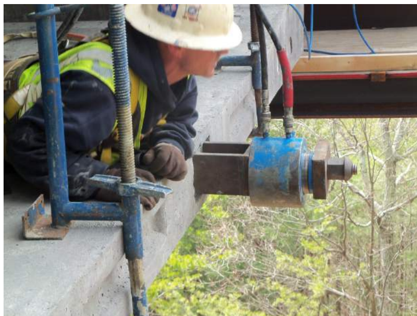
Figure 1.36 - Stressing Temporary Bar in Bottom Slab of the Foothills Parkway Bridge No. 2
