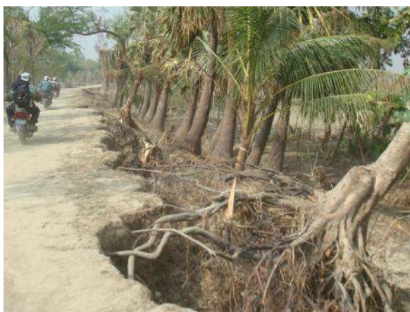
Figure 2.4: Failure of embankment due to overturning or uprooting of trees during cyclone (Mohammad Shariful Islam, BUET)
