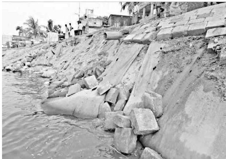
Figure 2.7: Poor performance of CC blocks at Keraniganj Beribadh site (Source: Prothom Alo, dt: 04.04.2011)
