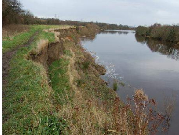
Figure 2.3: Photograph showing failure of embankments due to turbulent water currents (Wikimedia Commons, 2010)
