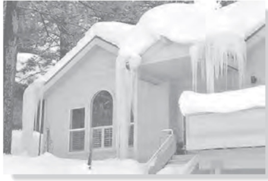
Excessive snow and ice loadings act on this roof.
