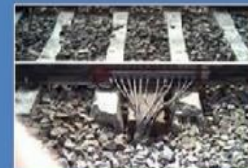
Wheel Impact load detection system
