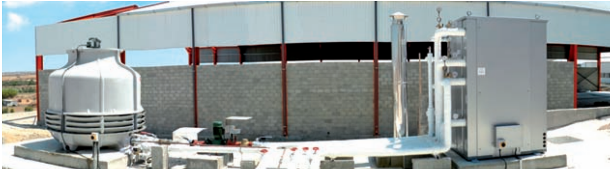
Figure 4.4: First solar airconditioning system in Cyprus, L' Amor Rouge Bakery
