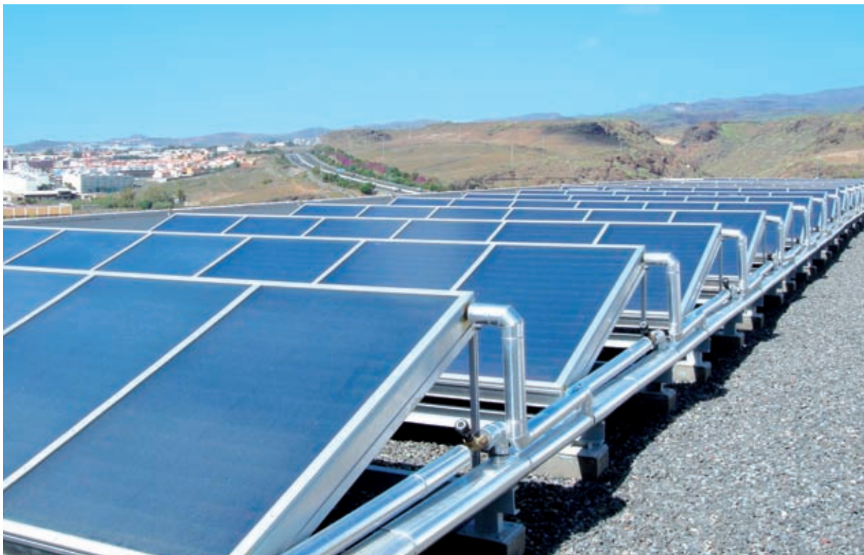
Figure 3.1: Solar Cooling installation
