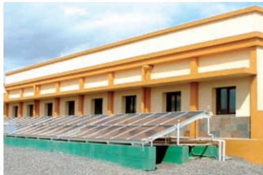
Figure 4.1: Solar collector field
