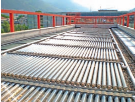
Figure 4.7: Solar vacuum tube collectors installed on EURAC roof
