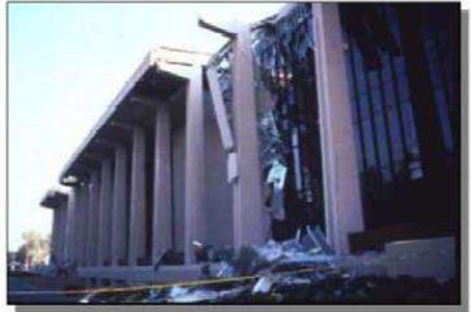
Exterior damage to the back (north side) of Oviatt Library during Northridge Earthquake (attributed to pounding).
