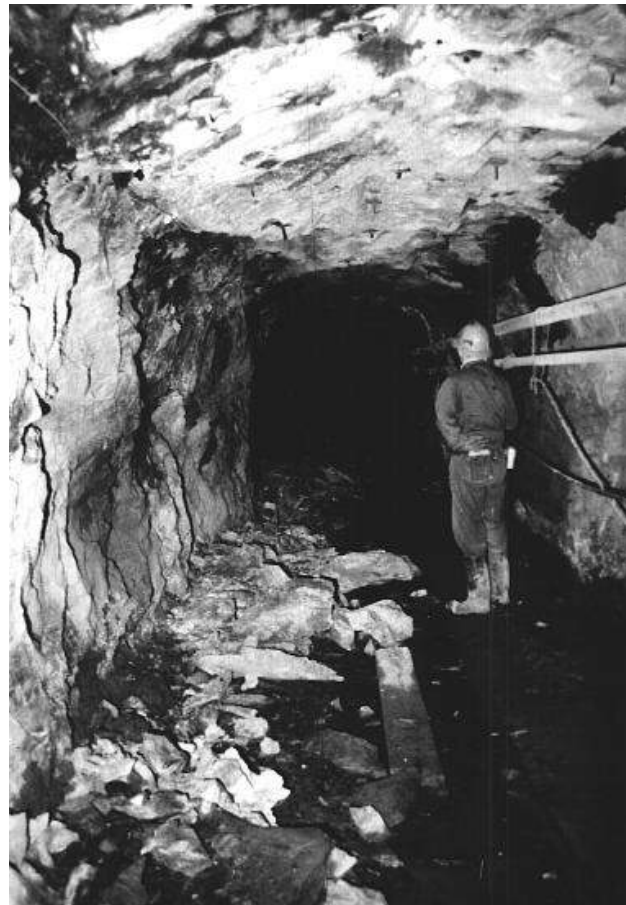
Figure 10.2: Spalling of one wall of a drive in quartzite at a depth of about 1,500 m in a uranium mine. In this case, an open stope on the left of the picture caused the stresses in the left-hand wall of the drift to be high enough to initiate spalling. This spalling is relatively minor and is parallel to the drift wall.
