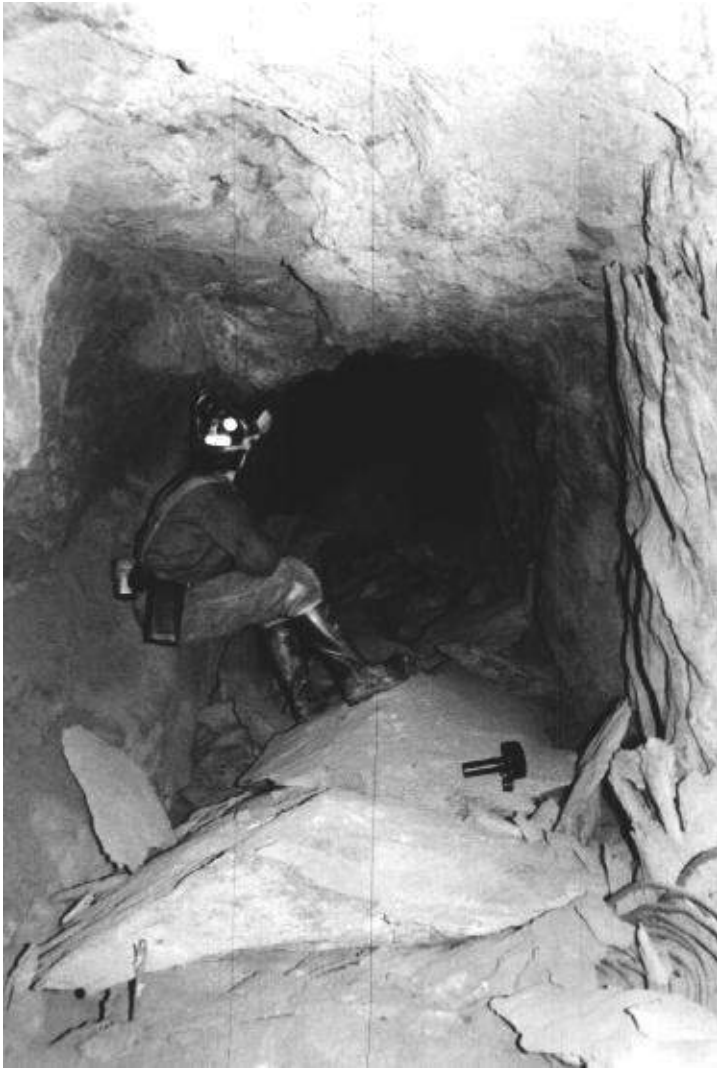
Figure 10.3: Spalling from the roof of an opening in highly stressed rock. The slabs on the floor have come from the left-hand side of the roof, just above the man's head. Spalling parallel to the right-hand sidewall is also visible.
