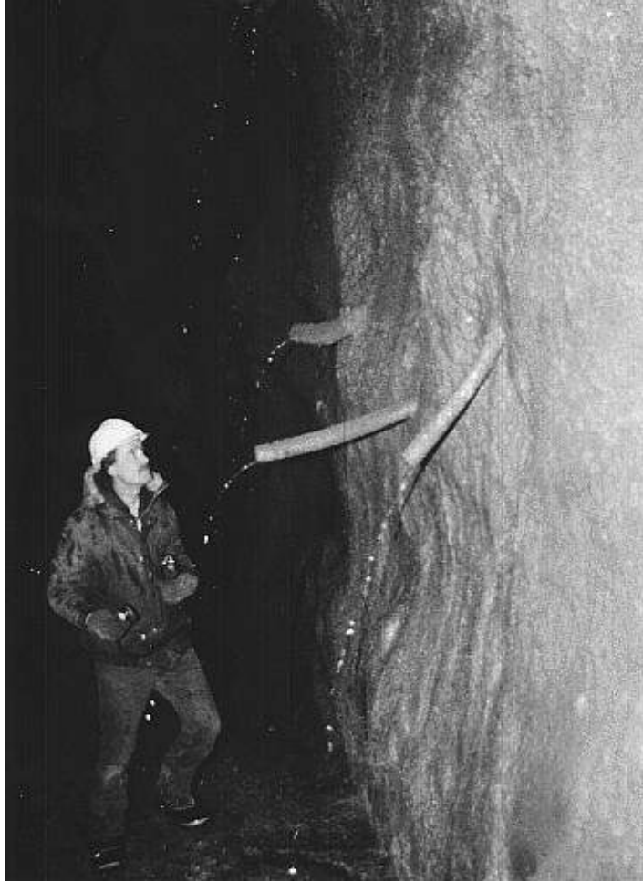
Figure 15.9: Plastic pipes used to provide drainage for a shotcrete layer applied to a rock mass with water-bearing joints.
