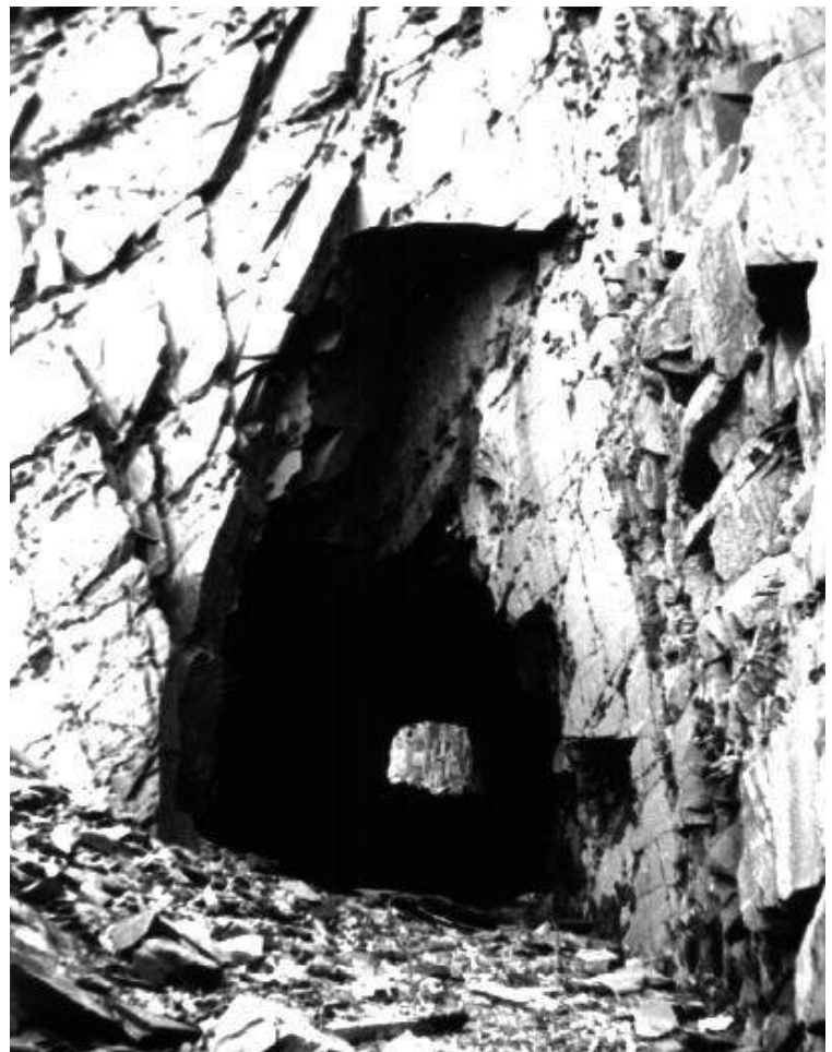
Figure 11.10: Structurally controlled failures in an old slate quarry in Wales. No support was installed in this tunnel and the final profile is defined by the wedges which have fallen from the surrounding rock mass.
