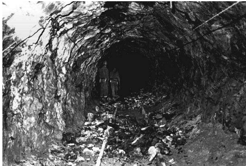
Figure 6.5: Ravelling of small wedges in a closely jointed rock mass. Shotcrete can provide very effective support for such rock masses.
