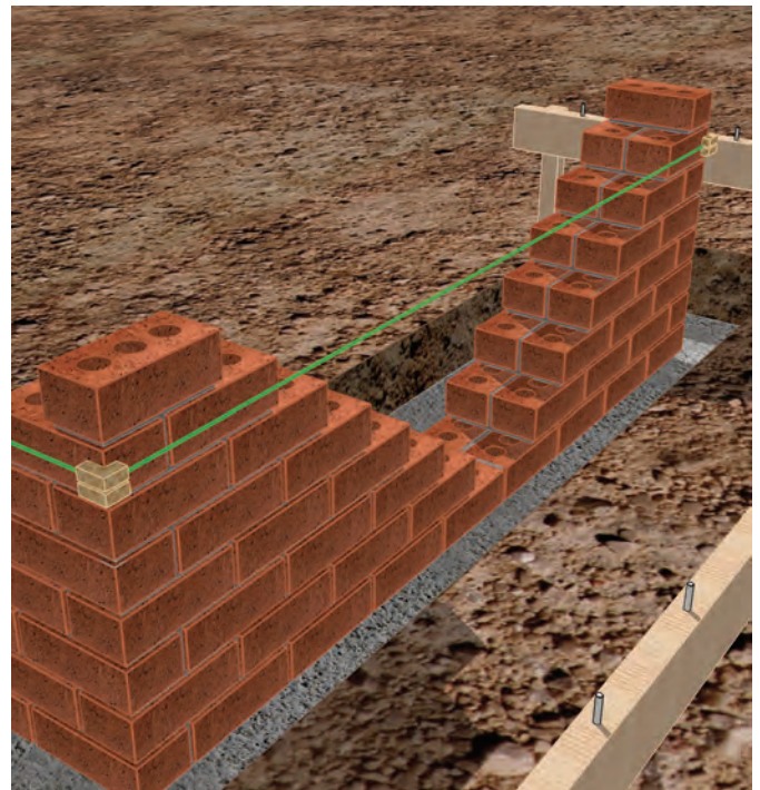
11.15 - Filling in the brickwork between corners, a builder's line and line-blocks or line-pins are used to ensure that each course is laid straight.
