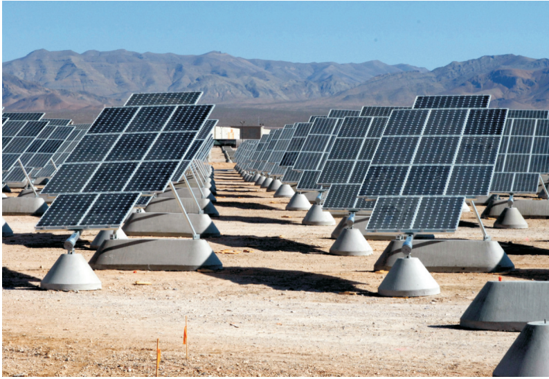
Fig. 7. Solar array at Nellis Air Force Base. These panels track the Sun in one axis. Credit: U.S. Air Force photo by Senior Airman Larry E. Reid Jr. http://upload.wikimedia.org/wikipedia/commons/d/de/Nellis_AFB_Solar_panels.jpg
