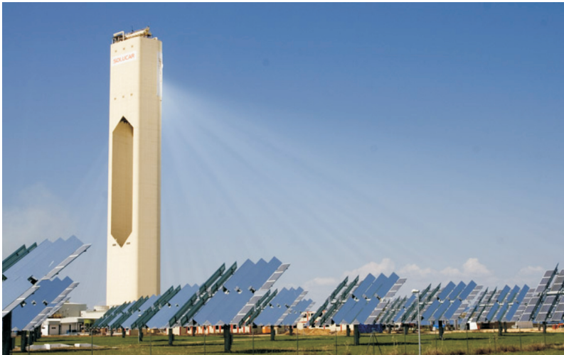
Fig. 17. The PS10 concentrates sunlight from a field of heliostats on a central tower. Credit, afloresm. http://upload.wikimedia.org/wikipedia/commons/e/eb/PS10_solar_power_tower.jpg
