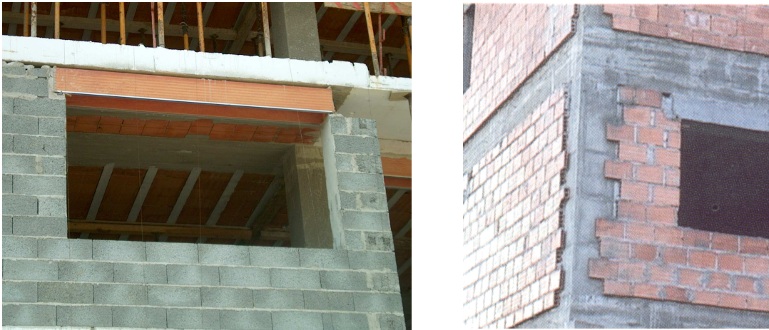
Figure 16: Examples of defects and masonry wall enclosure pathology
