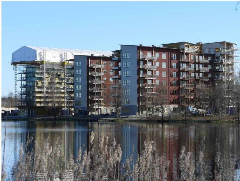
Figure 1 - Limnologen, eight storey residential buildings with timber structure in Växjö, Sweden. To the left, still under construction with a shield for weather protection. (Photo: Växjö University)
