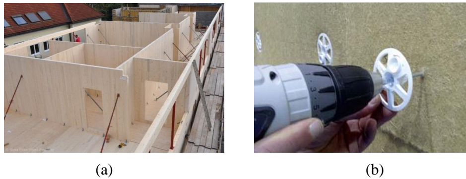
Figure 7 – Building with cut-to-size CLT elements; (a) CLT wall panels erected; (b) Fixing the wood fiber insulation panel to the CLT wall with special screws and a plastic washer.
