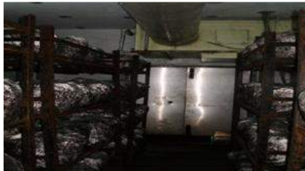
Fig. 11.26 Air handling unit inside the cropping room
