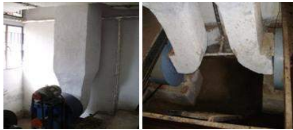
Fig. 11.24 The blowers fitted near the pasteurization chambers for circulation of fresh air and steam
