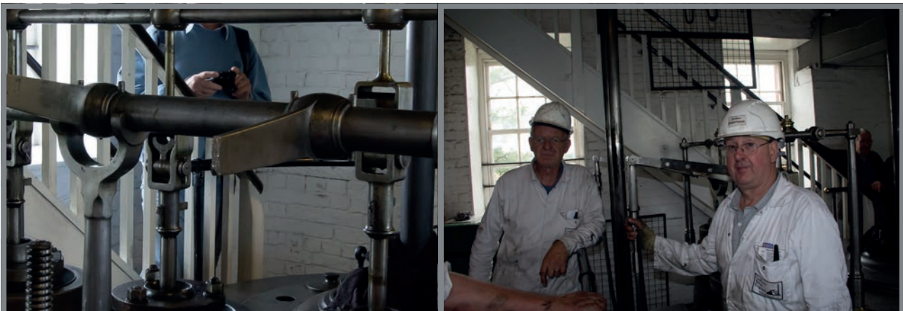
Throttle arm breakage on the Boulton & Watt No.1 engine Crofton Pumping Station, July 2017. This occurred early in the start process and no further damage was caused to the engine. A temporary repair was made to enable operation to be resumed, pending professional conservation advice on permanent repair. This incident was an opportunity to review and improve inspection, maintenance operational and safety procedures, along with conservation and recording practices.
