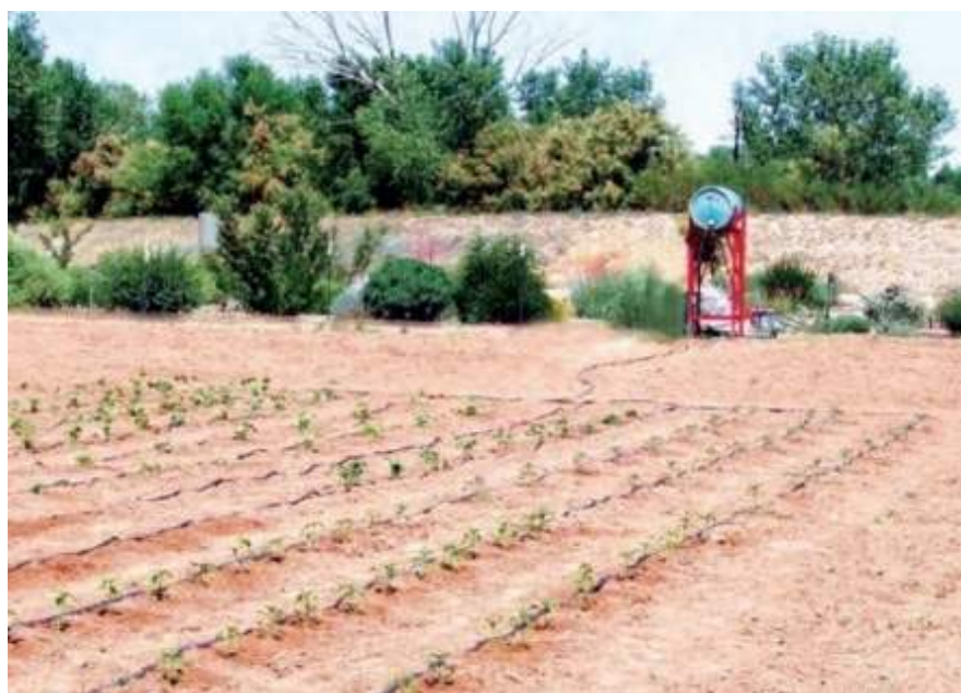
Figure 14.6. Example of an arrangement at the control station for a microirrigation system.
