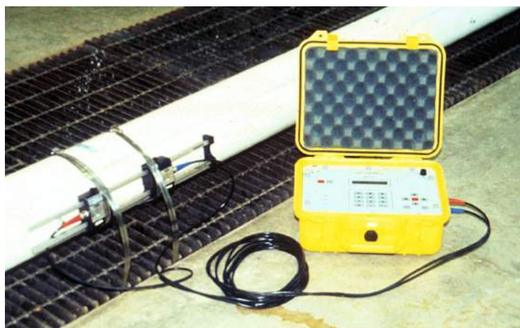
Figure 3.13. Clamp-on ultrasonic meter installed on a pipeline.
