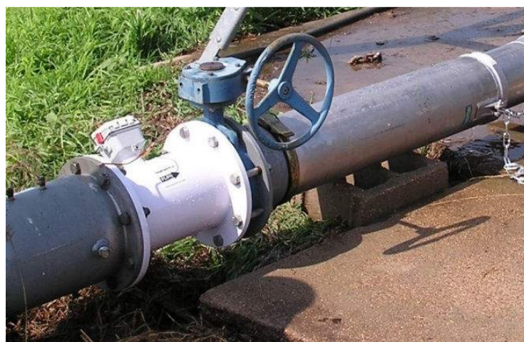
Figure 3.15. Electromagnetic flowmeter installed in the field.
