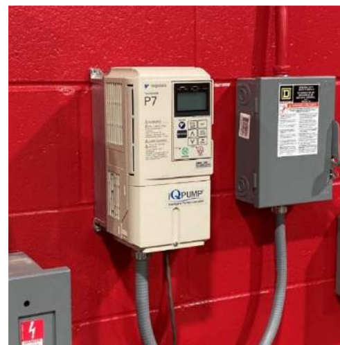
Figure 8.16. Panel for a variable frequency drive (VFD) electric motor controller.
