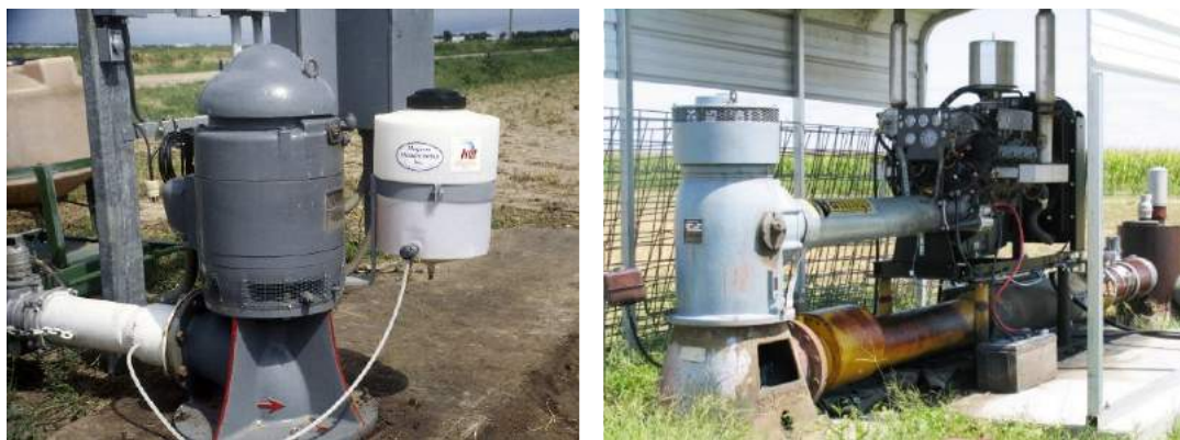
Figure 8.15. Pumping plants including a well with a vertical turbine pump and a power supply: electric motor (left) and internal combustion engine (right).
