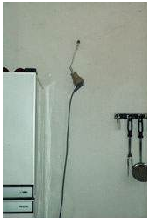
Dangerous electrical wiring, fire waiting to happen.
