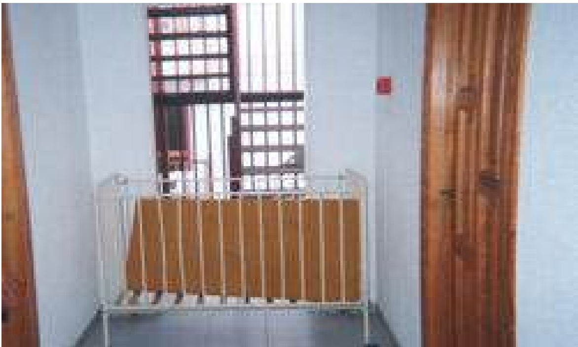
Blocked Fire Exit. Death trap.
