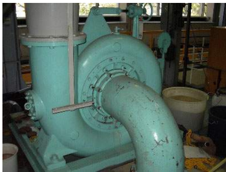
(a) Francis turbine
