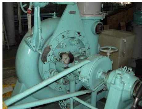
(b) Francis turbine from other side
