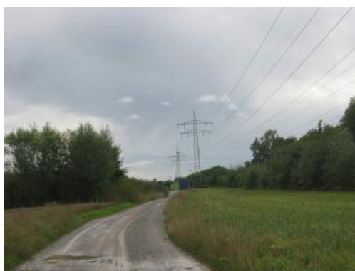
FIGURE 24.9 This high-voltage traction power line running to Eutingen Railway Substation in Germany radiates electromagnetic waves with very long wavelengths. (credit: Zonk43, Wikimedia Commons)
