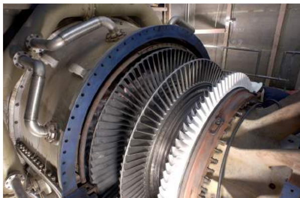
FIGURE 23.23 Steam turbine/generator. The steam produced by burning coal impacts the turbine blades, turning the shaft which is connected to the generator. (credit: Naponaco, Wikimedia Commons)
