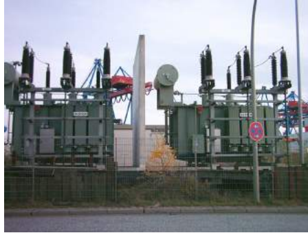
FIGURE 20.17 Power is distributed over large distances at high voltage to reduce power loss in the transmission lines. The voltages generated at the power plant are stepped up by passive devices called transformers (see Transformers ) to 330,000 volts (or more in some places worldwide). At the point of use, the transformers reduce the voltage transmitted for safe residential and commercial use. (Credit: GeorgHH, Wikimedia Commons)
