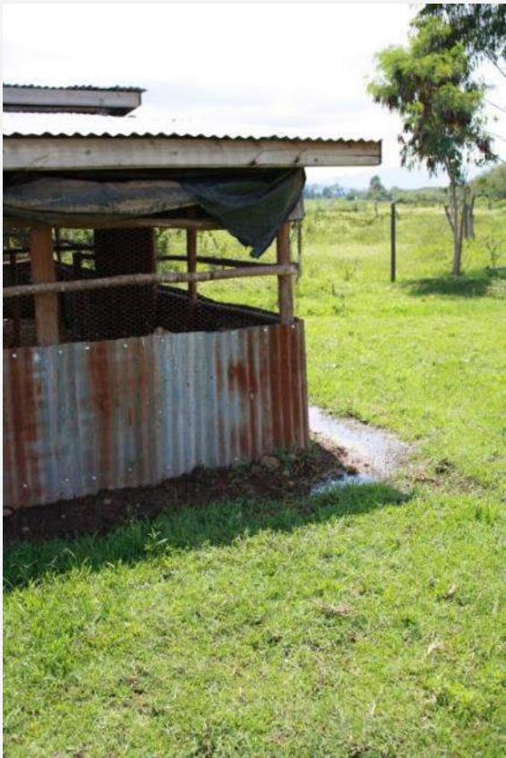
Poor storm water drainage
