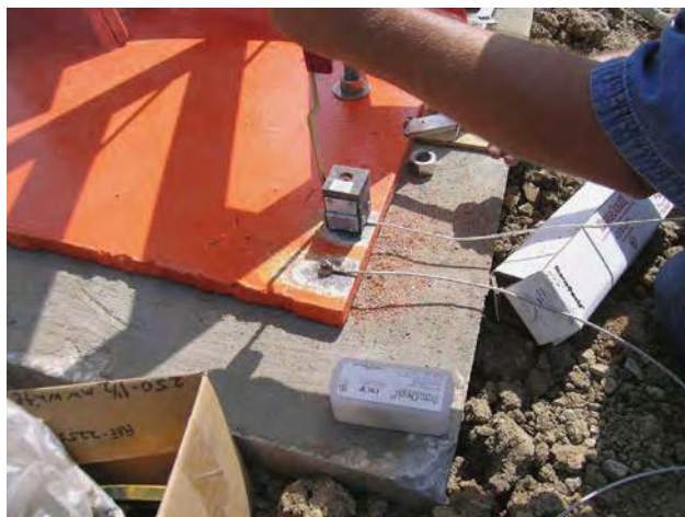
Figure 11a A thermite explosive charge is used to produce an extremely high temperature that bonds the cables instantly to the sculpture's clean metal surface.
