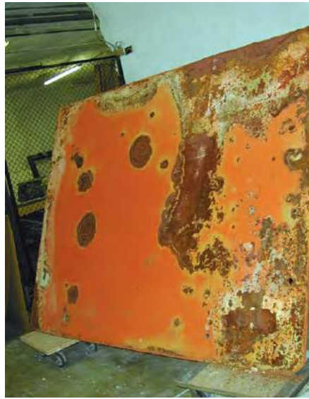
Figure 9 (Right) Bottom surface of the base plate, showing heavy rust and missing paint. (Far right) Detail of the contact area between steel beams, showing heavy rust and missing paint.
