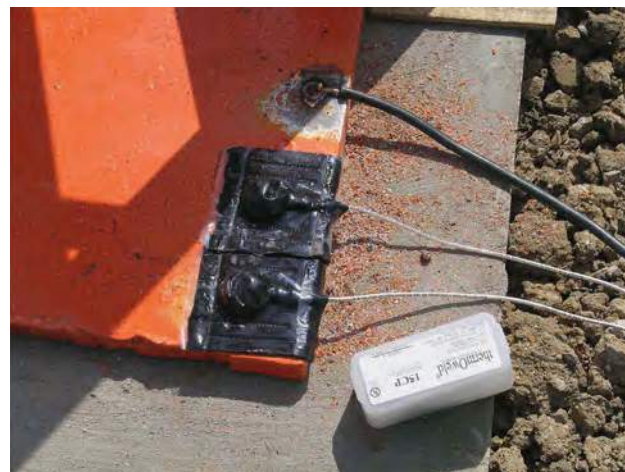
Figure 11b The cable connections to the sculpture are coated with a bituminous material to make them waterproof.
