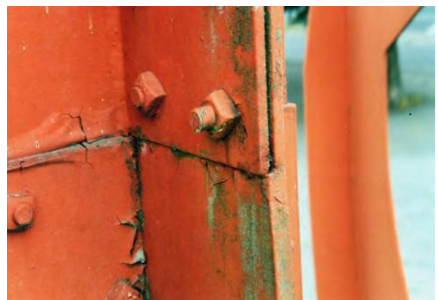
Figure 6 Photo of the west-facing side, showing gaping or open joints where a nut had not been tightly fixed. Loss of paint included flaking of the top layer or several layers, down to the primer. © 2014 Calder Foundation, New York / Artists Rights Society (ARS), New York. © ZMK, Hannover 2003.
