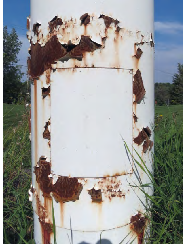
Figure 3 Example of deterioration due to improper maintenance, showing paint lifting and corrosion of steel behind the weeds. Photo: Marie-Chantale Poisson, 2012 © CCQ.
