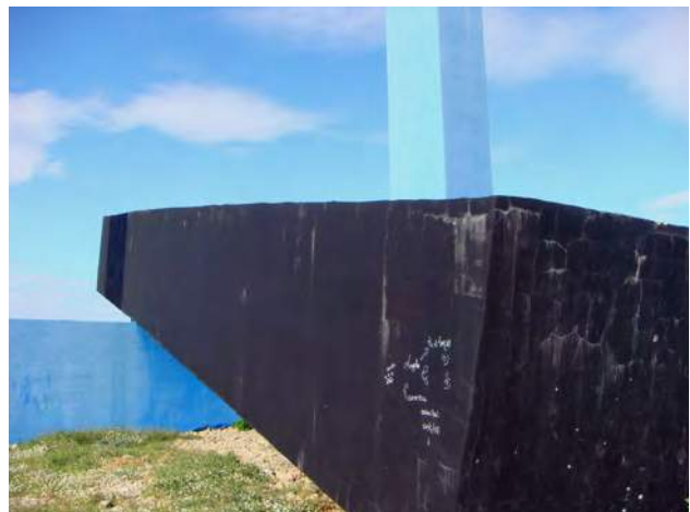
Figure 5 Detail of a work by Tano Festa, showing damage to the black latex paint on concrete from light exposure, rain, and graffiti. Tano Festa, Monumento per un Poeta Morto , 1989 (detail). Situated in Fiumara d'Arte, Sicily. Courtesy Fondazione Fiumara d'Arte. Photo: Tom Learner.
