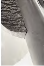
Figure 3 Crack between an aluminum quill and a fiberglass feather observed on one of the Shuttlecocks shortly after their 1994 installation.
