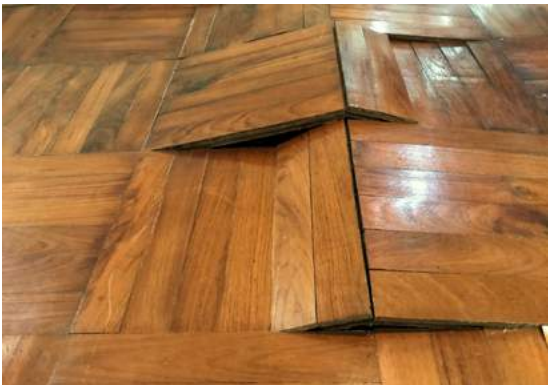
Fig.07/29 Moisture content of the environment causes the wood to expand and contract.
