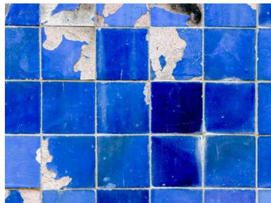
Fig.08/20 The layer of glaze on ceramic tiles is actually thin, can crackle and wear off over time.
