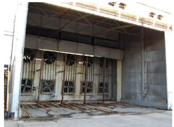
Fig.07/28 Lumber drying kiln.
