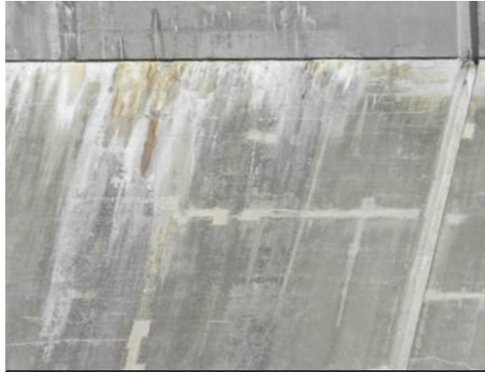
Fig.06/03 Efflorescence refers to the white salt stains indicating significant moisture exposure.
