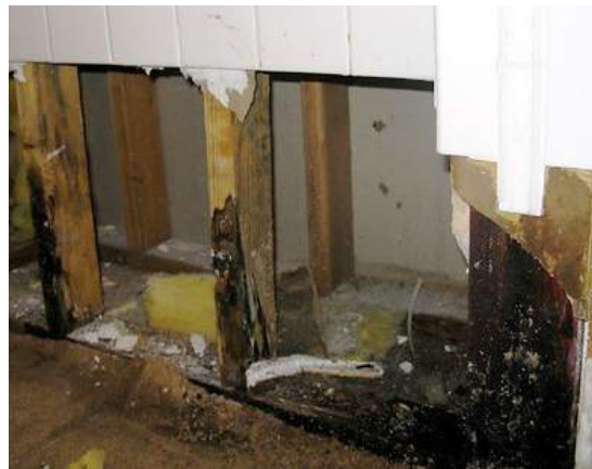
Fig.01/13 Water can easily cause destruction behind wall finishes, without the occupants ever noticing.
