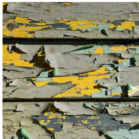
Fig.03/14 Flaking lead paint particles create serious health risks.
