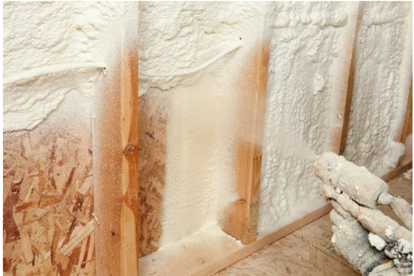
Fig.11/20 Polyurethane spray-foam insulation is highly efficient but requires flawless installation to properly function.
