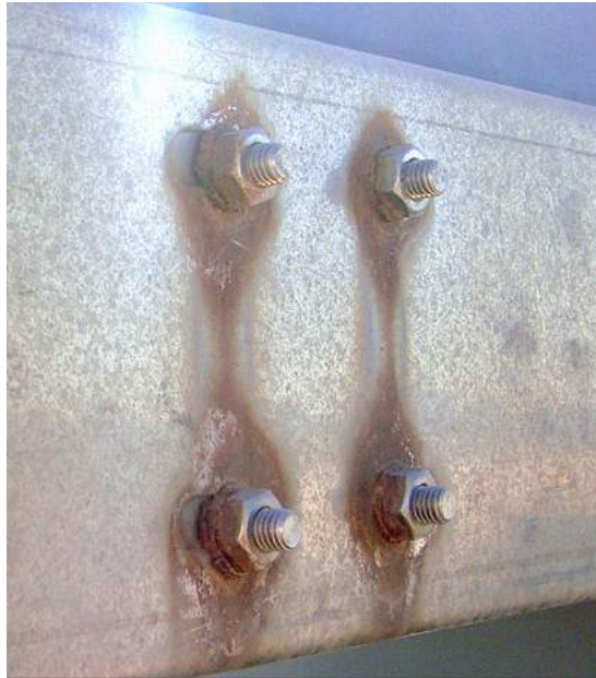
Fig.10/03 Galvanic corrosion can even happen between stainless steel (nut&bolt) and mild steel (beam).
