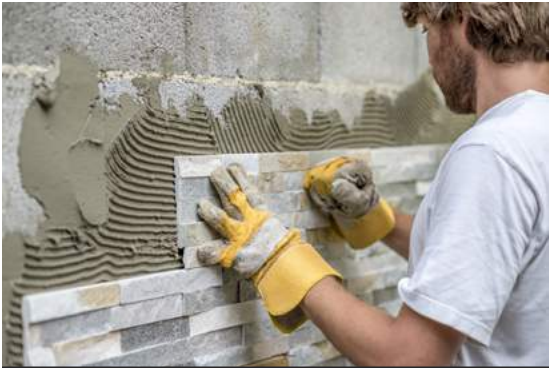
Fig.06/25 Natural stone veneers are being thinset on CMU (Concrete Masonry Unit) wall.
