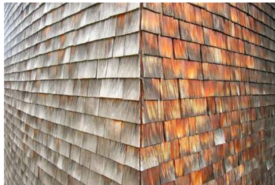
Fig.07/09 Wood shingles on different facades clearly depict the weathering effect of UV exposure.
