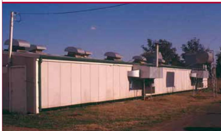
Oil or gas-fired hot air brooder units on side of shed for whole-house brooding: the entire brooding area is heated to the required temperature
