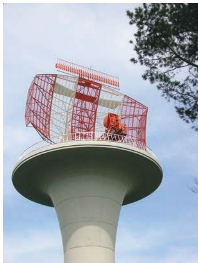
(a) Radar antenna. The parabolic antenna is the PSR and the rectangular one above it is the SSR. © Magnus Manske / Wikimedia Commons / CC-BY-SA-3.0.
