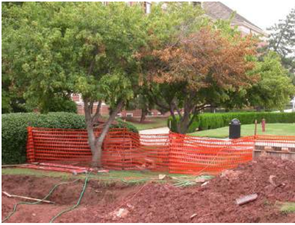
Figure 6.53. Damage to trees from construction and excavation of soil too close to the tree.
