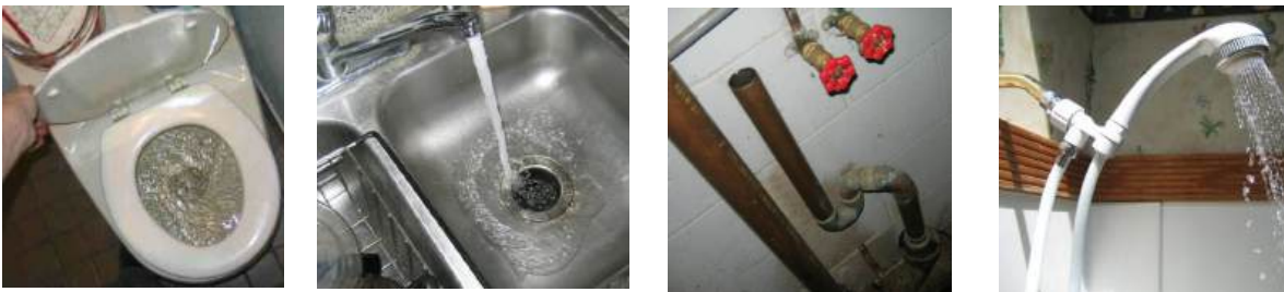
Pictures of various plumbing components and conditions provided by Ben Gromicko.
