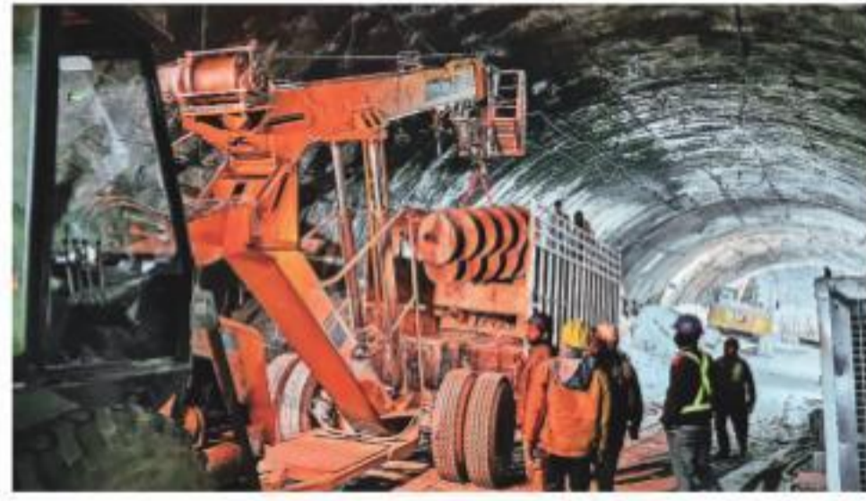
800-900 mm diameter MS pipes being inserted through the rubble inside Silkyara tunnel to prepare an escape passage for trapped workers in Uttarkashi district on Tuesday. PTI
