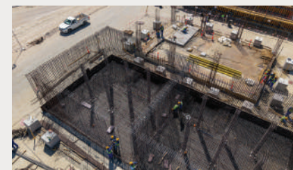
Irrigation Pump Station
