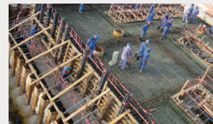
SW Pumping Station
