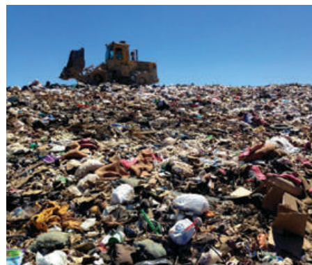
Bulldozer distributing waste at the Gila County landfill, Arizona, United States (Alan Levine).
