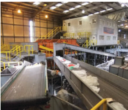
Material recovery facility for sorting mixed recyclables, London, United Kingdom (Urban Greendom).
