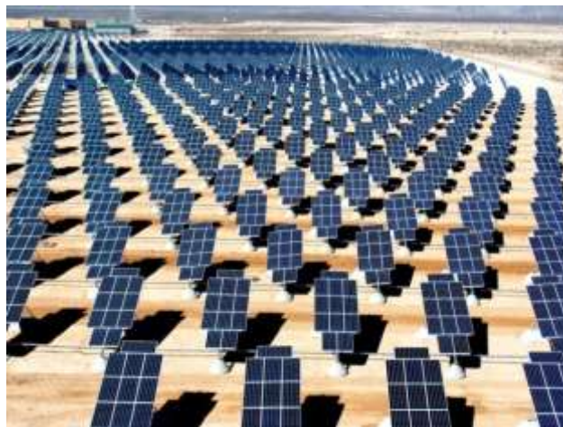
Fig. 7.15. PV Power Plant (source: U.S. Air Force, 2007)
