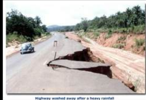
Highway washed away after a heavy rainfall
