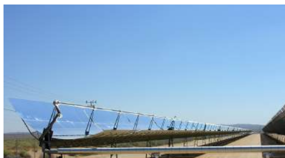
FIGURE 25.42 Parabolic trough collectors are used to generate electricity in southern California. (credit: kjkolb, Wikimedia Commons)
