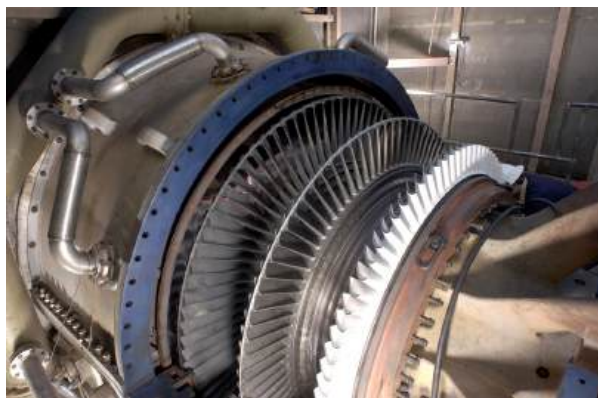
FIGURE 23.23 Steam turbine/generator. The steam produced by burning coal impacts the turbine blades, turning the shaft which is connected to the generator. (credit: Naponaco, Wikimedia Commons)
