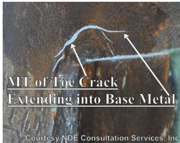
Figure 21: MT of toe crack
