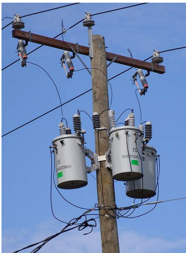
Figure 15.21 Transformers are used to step down the high voltages in transmission lines to the 110 to 220 V used in homes. (credit: modification of work by “Fortyseven”/Flickr)
