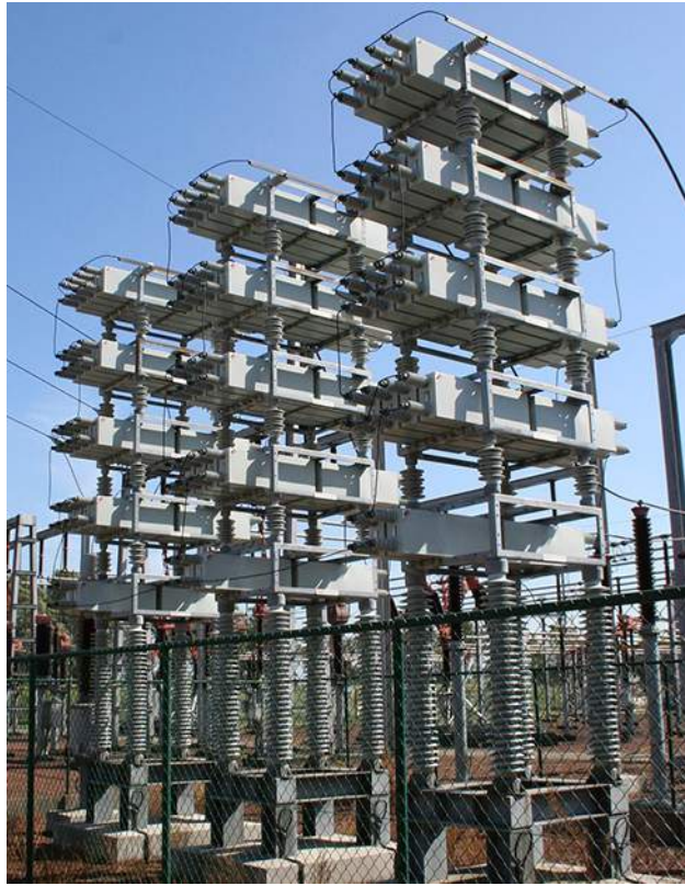
Figure 15.14 Power capacitors are used to balance the impedance of the effective inductance in transmission lines.
